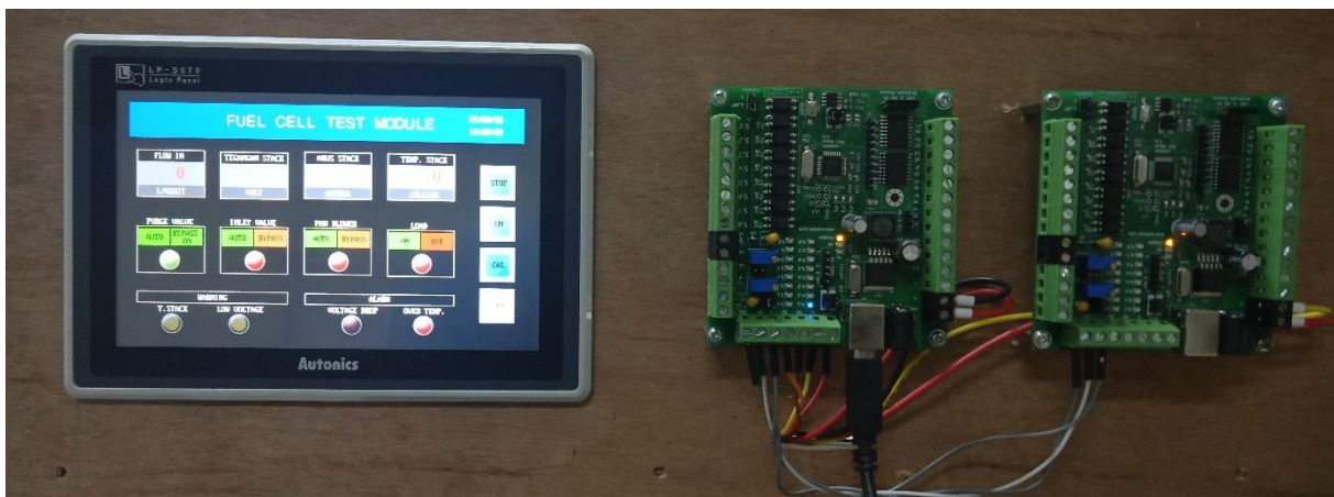
Figure 6. This picture shows HMI and two outseal plc installed modularly, one functions as a master and one as a slave so it has 4 analog inputs, 16 switches and 16 relay outputs. Communication between HMI and outseal PLC via RS232 port with Modbus RTU.
